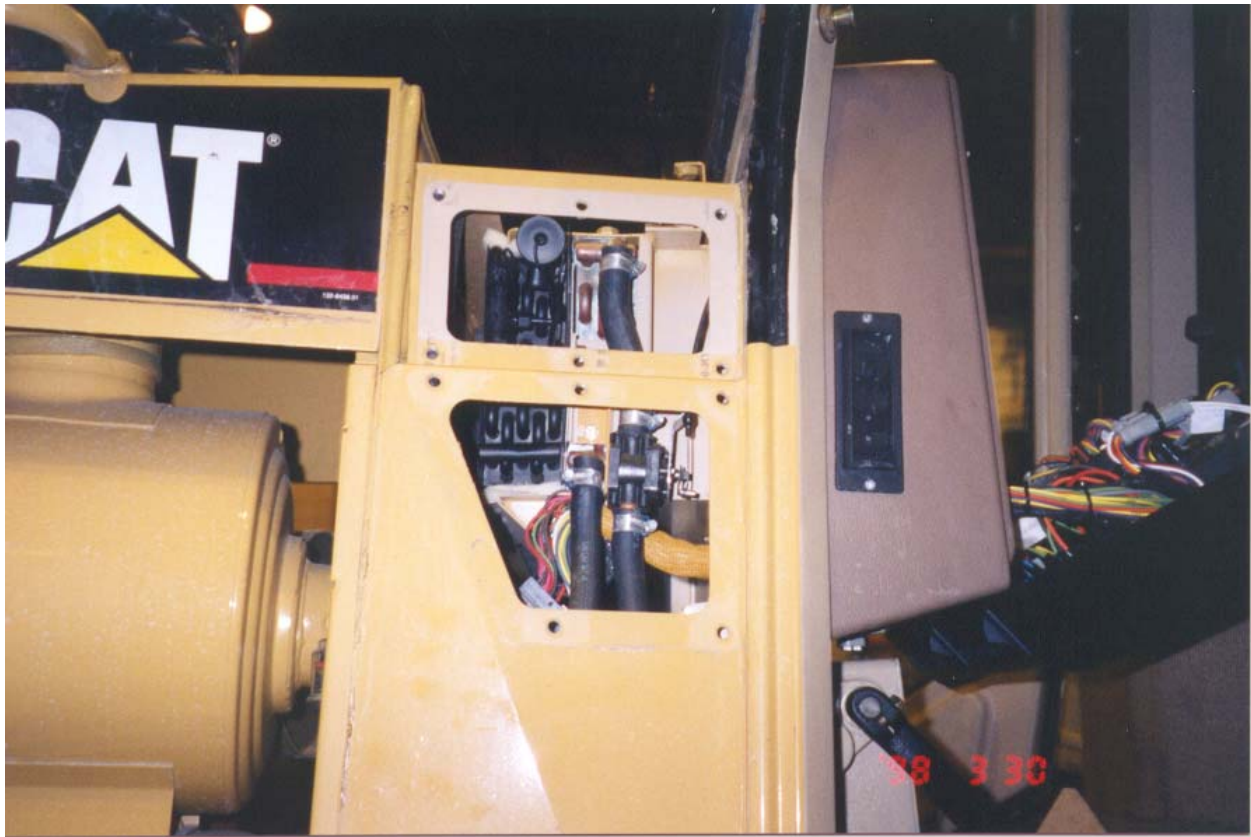
Evaporator in place alongside heater coil.
